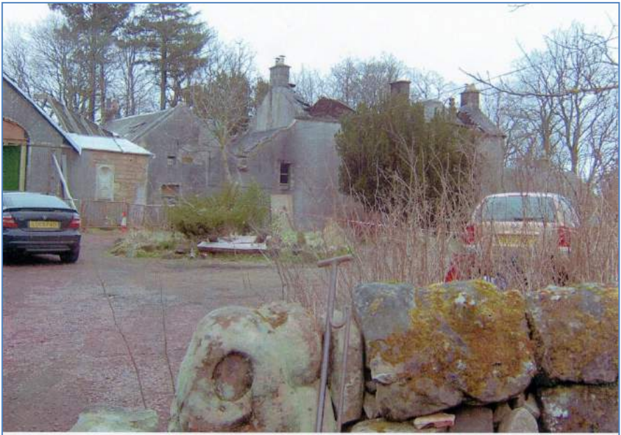
Badly damaged by fire in March 2016.
